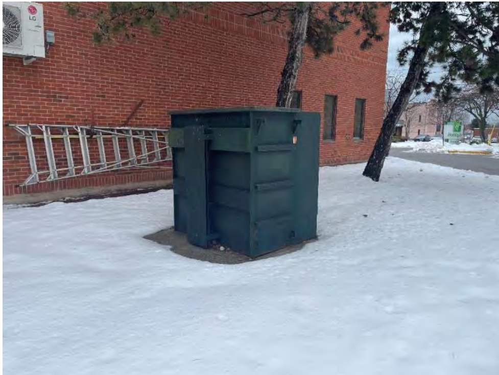
Photo 3: Transformer located on-Site to the west of the Site building, facing southeast.
