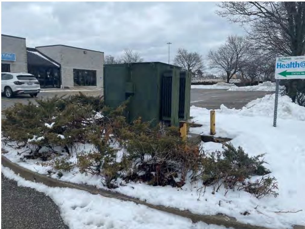
Photo 16: Transformer located at east adjacent property, 234 South Service Road East.
